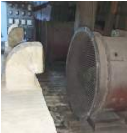
Hot Air Ducting
